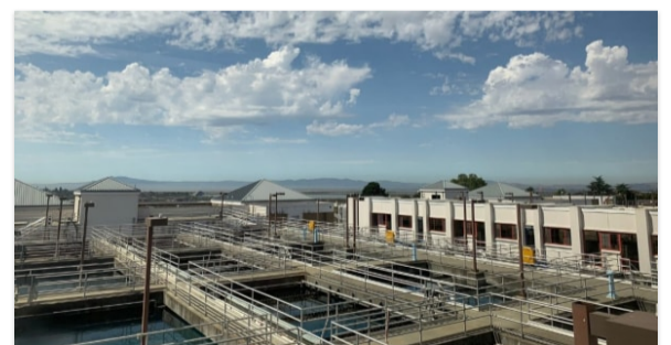
7,000 gallons of disinfectant discharged at Vallejo water treatment plant
